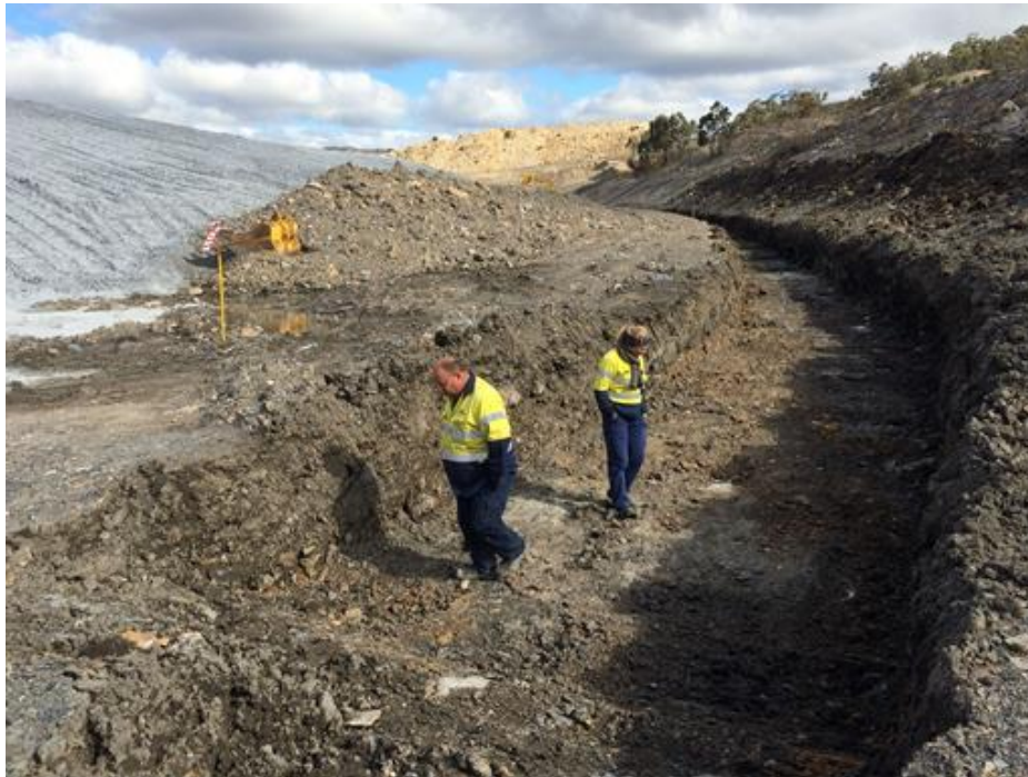
Plate 1 View south along the excavated Lamberts North drainage line circa 2014. Courtesy: Lend Lease
