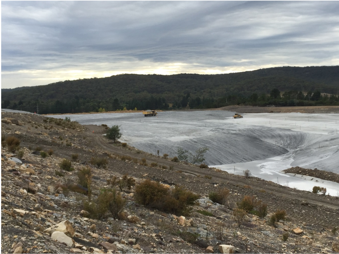
Figure 5 | Photograph of Lamberts North South eastern boundary with dump truck and dozer operating
