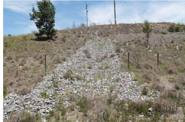
Water drop structure in treed area adjacent transect 8 in good condition and stable
