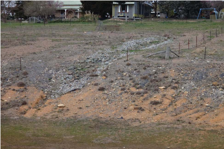
Figure 6 Minor erosion of sediment retention basin wall
