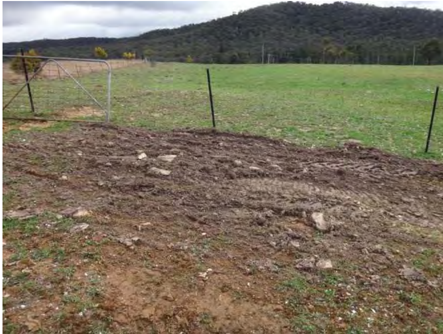
Plate 3 Soil settling hole repaired
