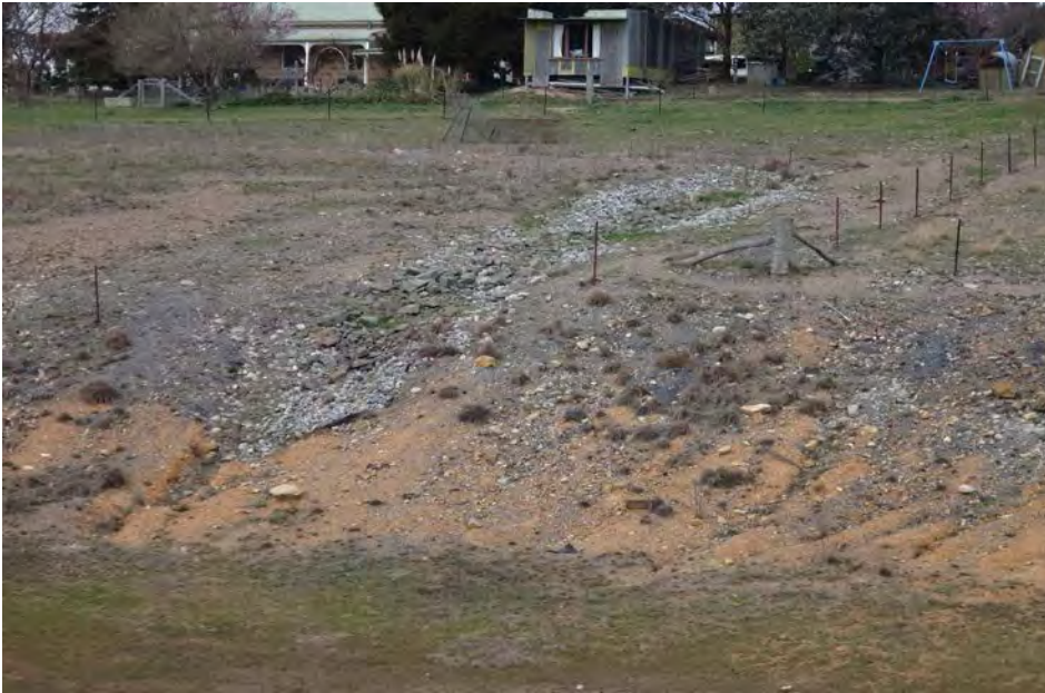
Figure 6 Minor erosion of sediment retention basin wall
