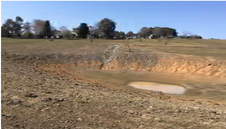
Figure 2 Indicative condition of sediment retention basins
