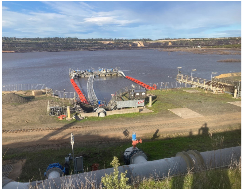
Figure 2: Fire Service Pump Infrastructure to Remove Water From the Mine to the Latrobe River
