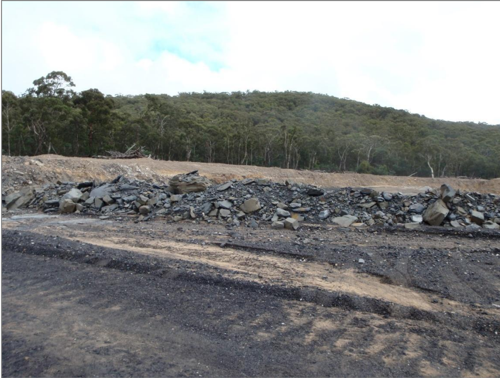
Plate 3: View west across proposed Lamberts South ash emplacement area. The ash will only be placed in the disturbed areas in the foreground and will not impact the remnant vegetated area in the background. Site 45-1-0218 is within the vegetated area beyond the limit of disturbance, but was not accessible at the time of survey. The Mine Manager has assured OzArk that the site remains intact as per the active CHMP for the site.
