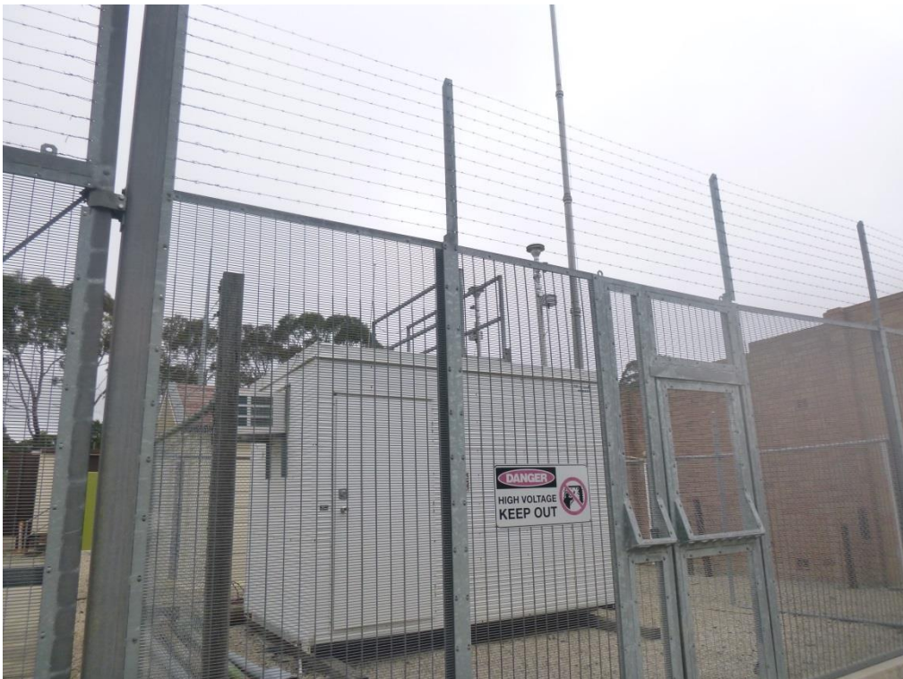
Photo 4 – Air Quality Monitoring Station (AQMS)
