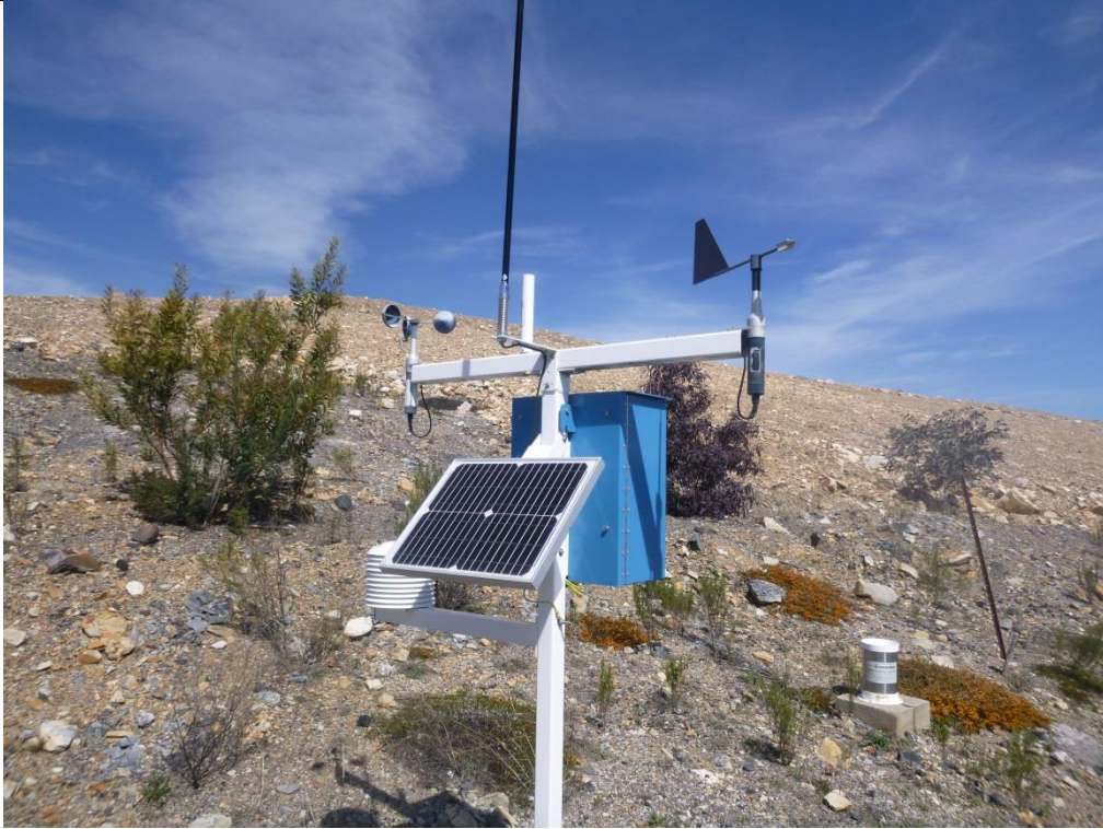
Photo 17 – Weather monitoring station at Area 1 repository
