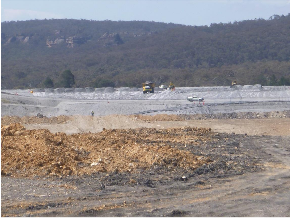
Photo 1 – Haul truck, roller, loader and light vehicle at the Lamberts North ash repository.
