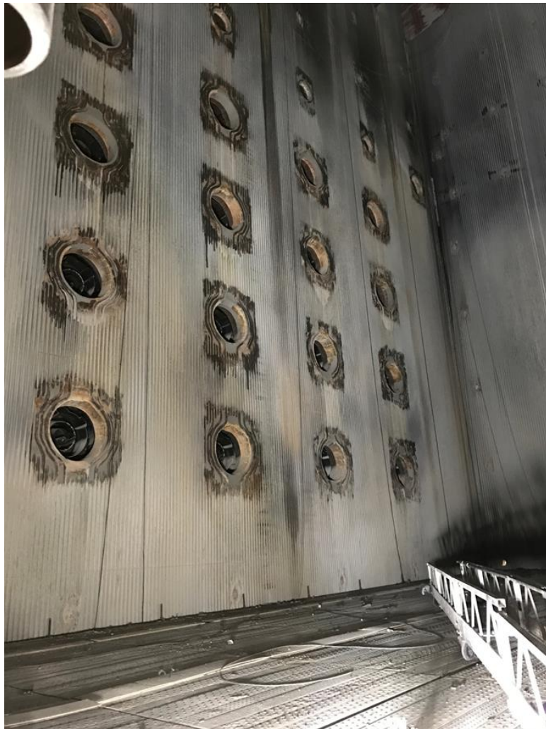
Inside one of Mount Pipers Boilers
