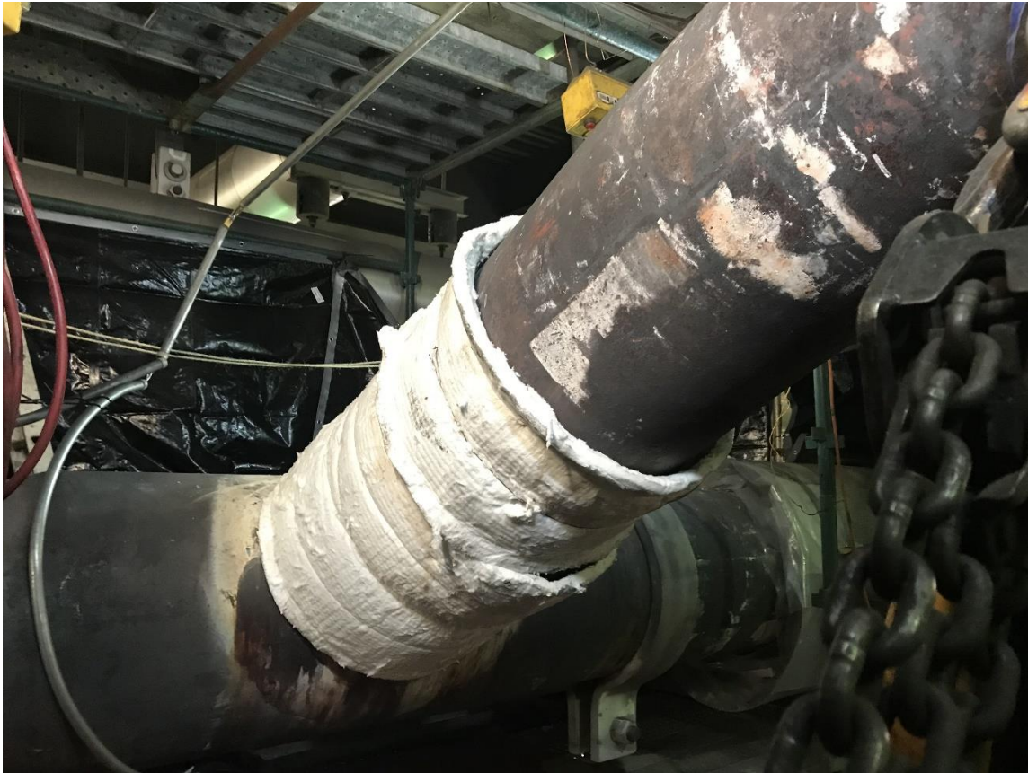
Steam Main with insulation removed
