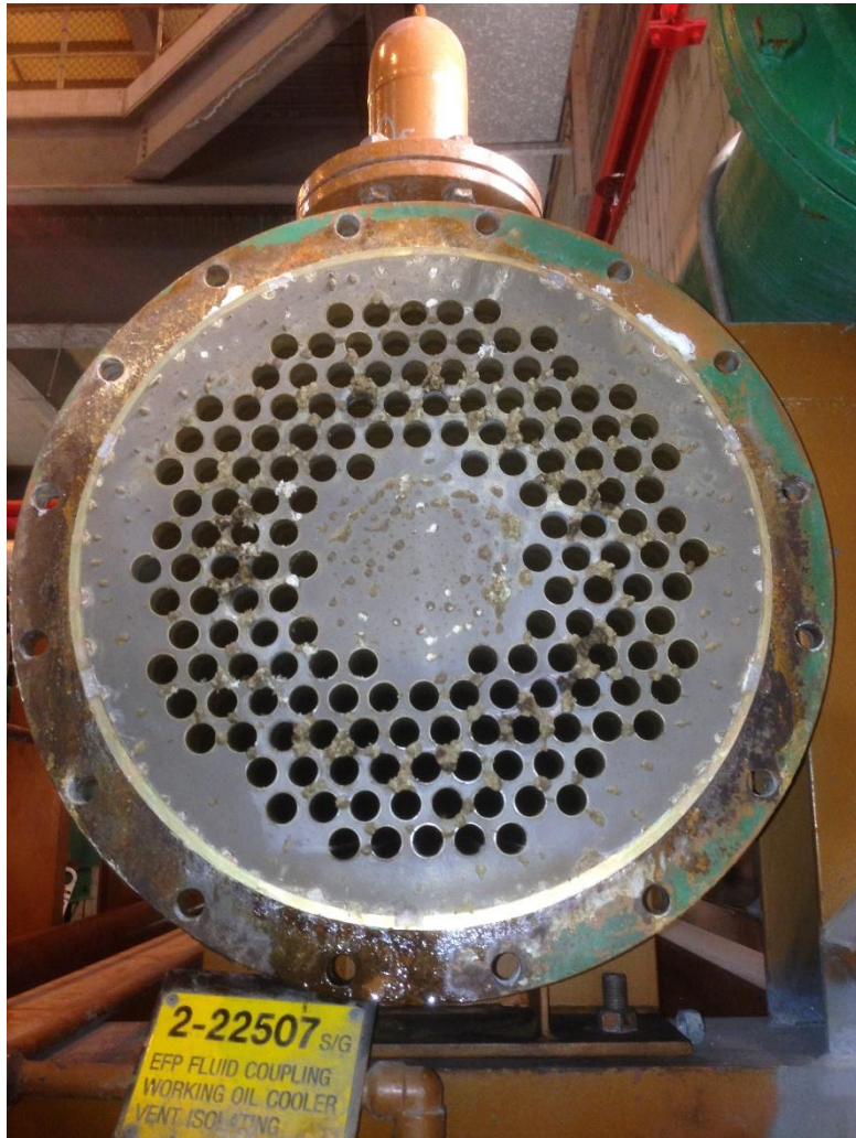
2 Electric Feed Pump Fluid Coupling Oil Cooler
