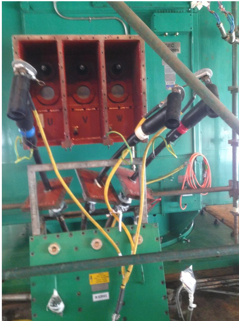
Motor Prepared for electrical testing
