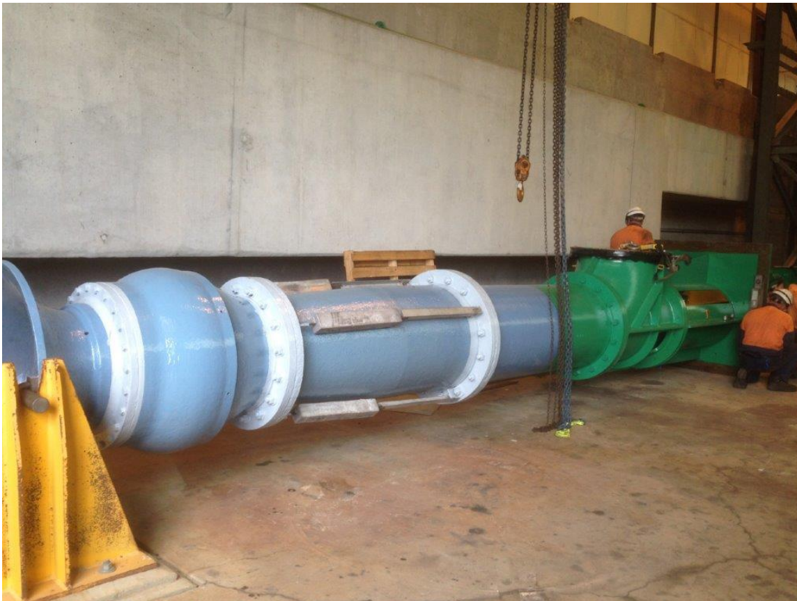
Overhauled Auxiliary Circulating Water Pump
