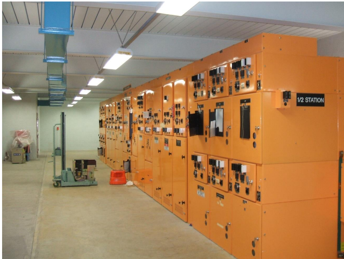
Typical Switchboard to be maintained
