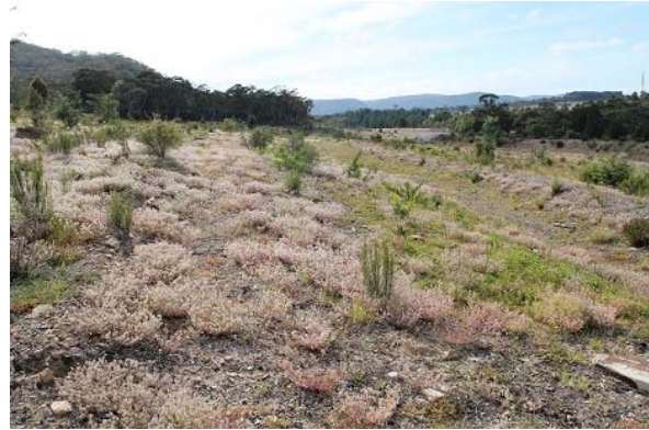
Area A: improved vegetative cover has improved the stabilisation of contour drains.
