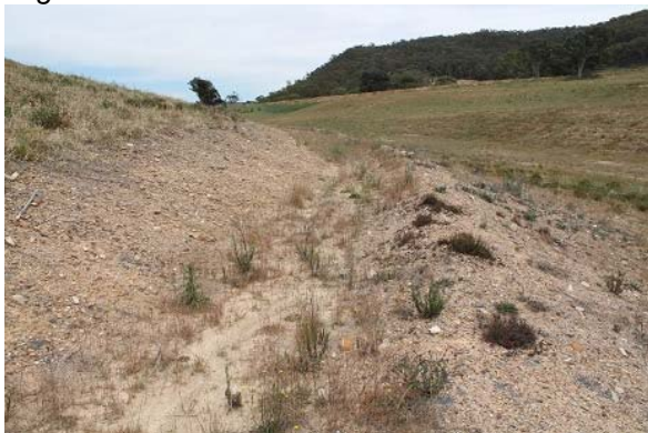
Area C: exposed contour drain subject to erosion and sedimentation with poor vegetative cover.
