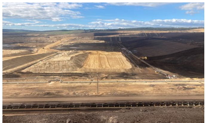
Strategic overheight dumping in Maryvale Field for coal coverage, weight balance against groundwater pressures, and buttressing coal batter adjacent Morwell River
