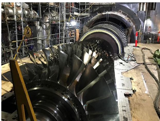
Figure 3-1: Existing turbine with cover removed
