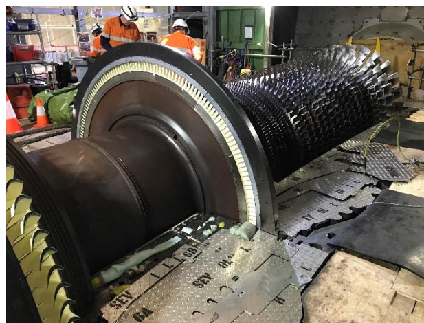
Figure 3-2: Existing turbine with cover removed
