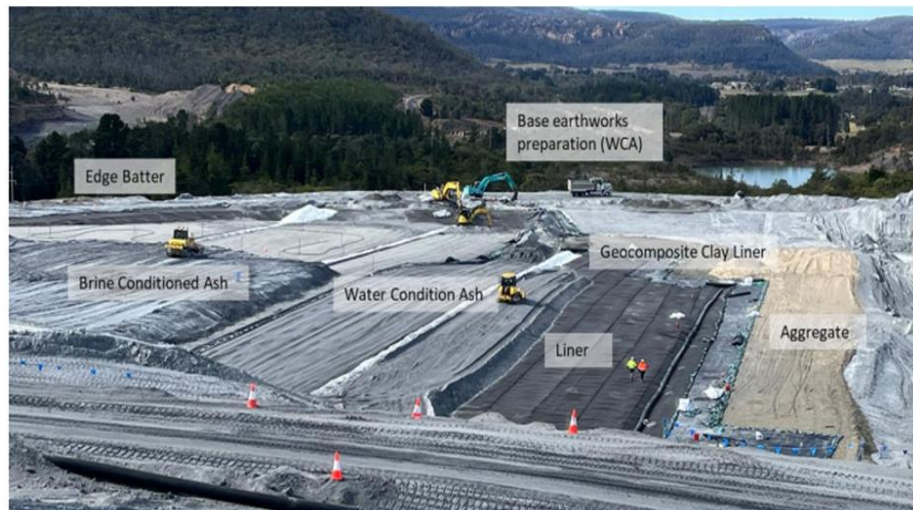
Plate 1 Installation of the leachate barrier in LNAR Stage 1A (Photo taken during Q3 2022)
